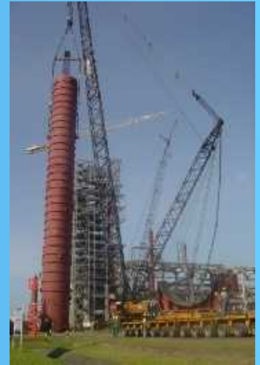
Installation for Deisohexanizer
