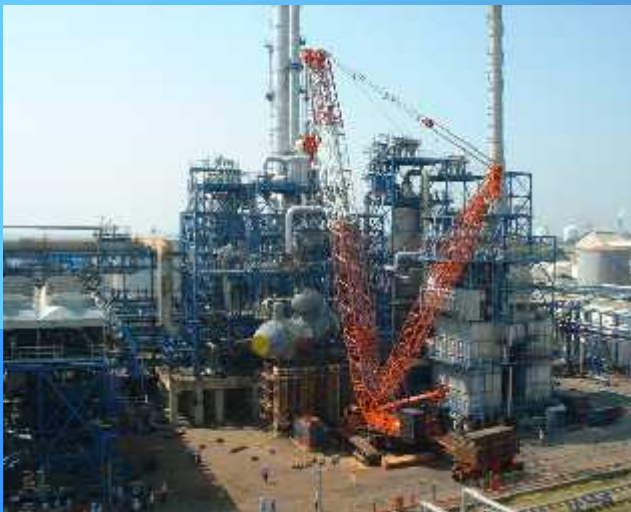
Replacement for Heat Exchanger
