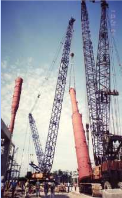
Installation for CO2 Absorber
