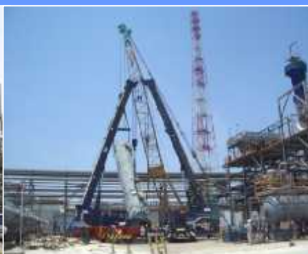
Installation for Amine Contactor
