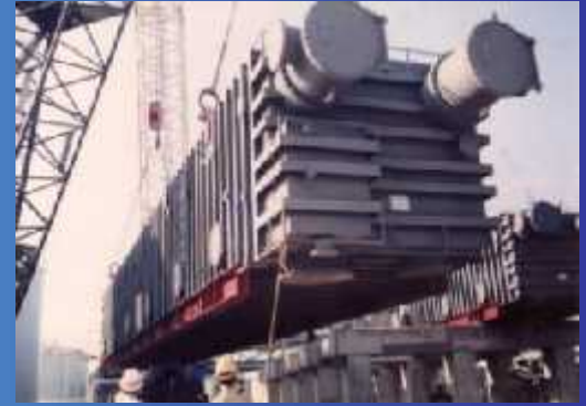
Installation for Desalination unit
