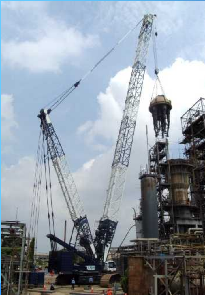
Cuting Shell Top Regenerator and Lift Down the Cover Include Cyclone Unit
