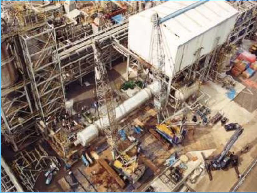
Replacement for Dryer
