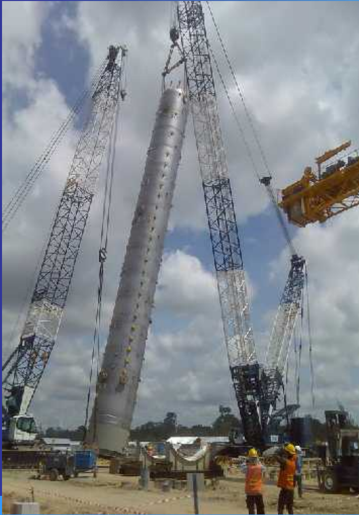
Installation for Absorption Tower
