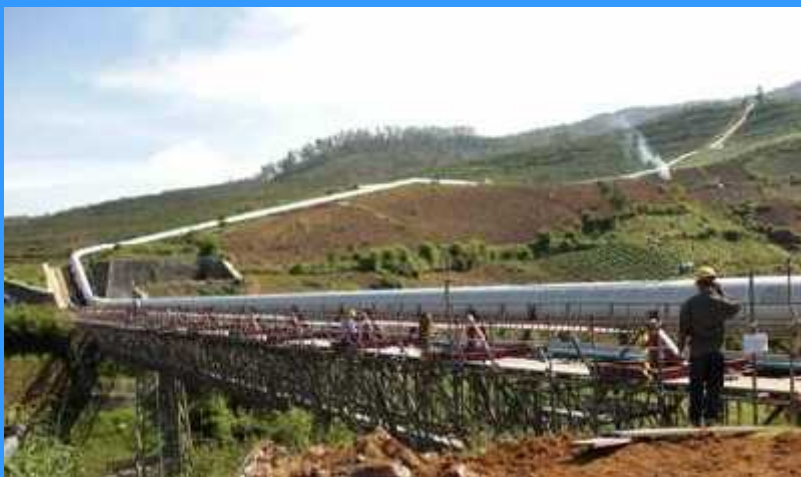
Pipe Line for Geothermal Power Plant
