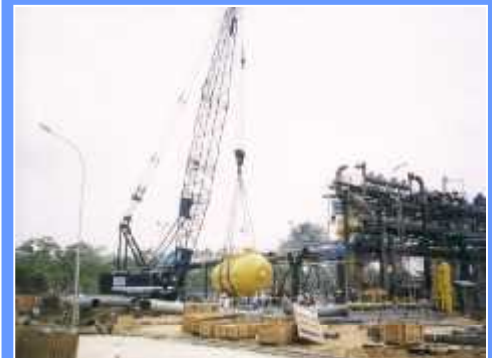
Installation for Slug Catcher
