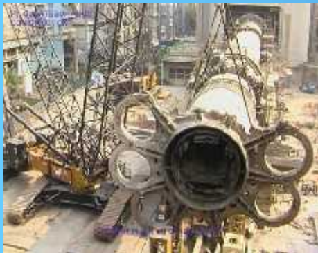
Installation for Shell Kiln
