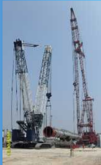
Installation for Deethylenizer
