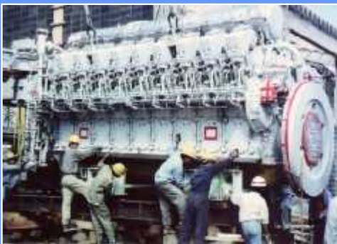
Installation for Engine Generator
