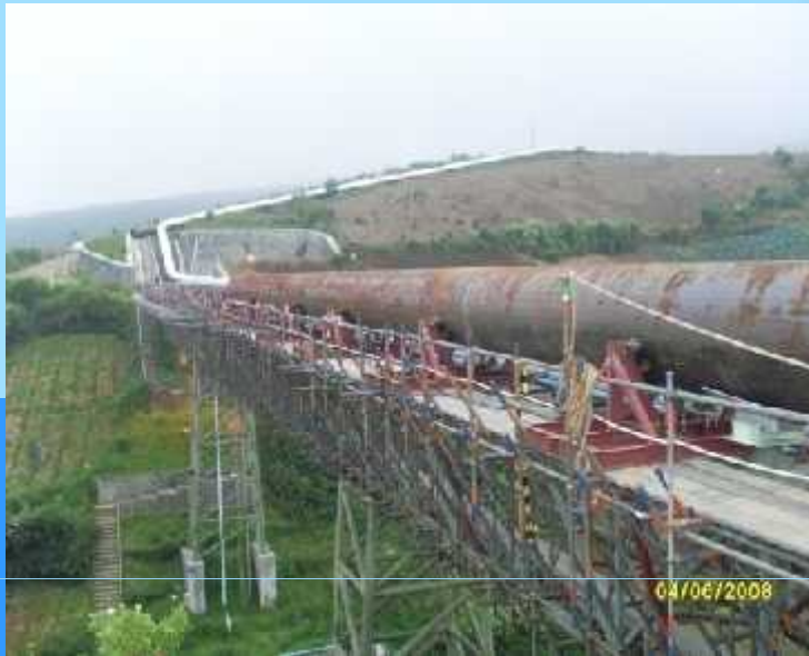
Pipe Line for Geothermal Power Plant
