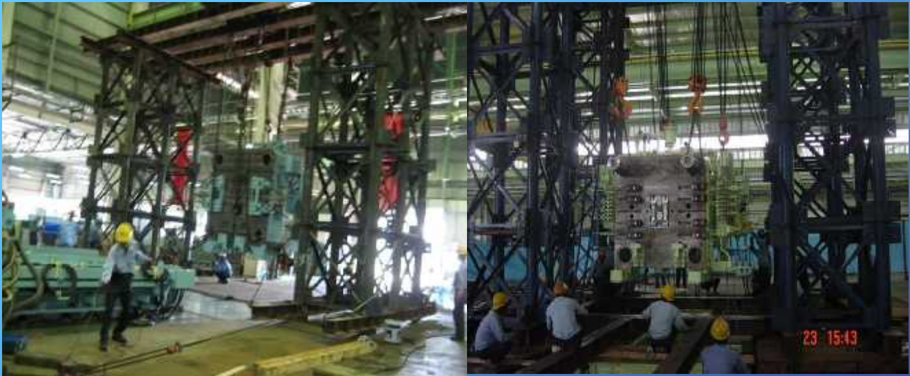
Installation for 1,250 Ton Die Casting Press Machine
