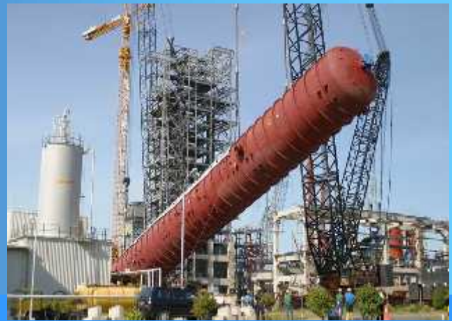
Installation for Deisohexanizer
