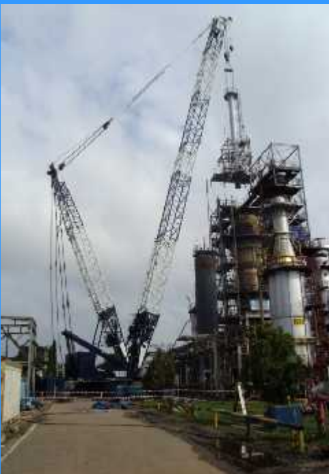
Replacement for Regenerator Stack
