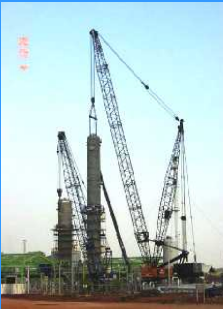
Installation for CO2 Absorber
