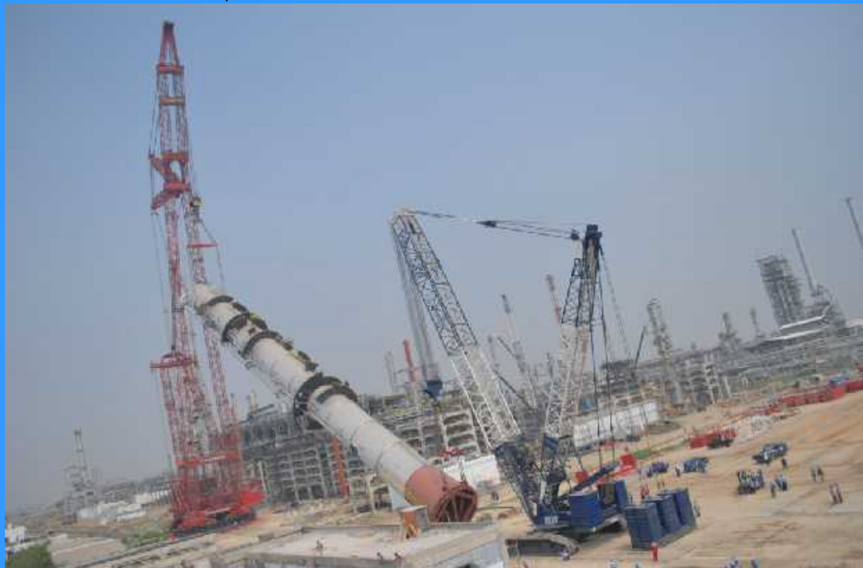
Installation for Deisohexanizer
