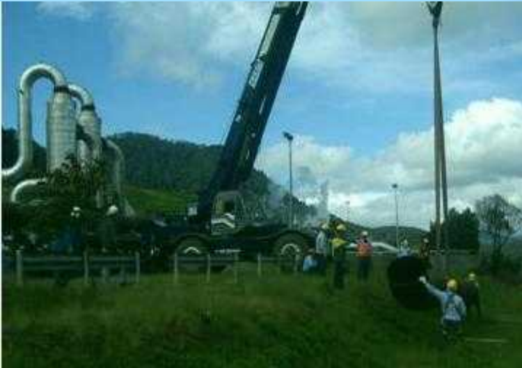
Pipe Line for Geothermal Power Plant
